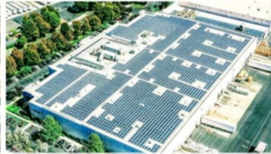
Synnex Corp. – 920kW
