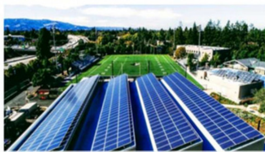
The Harker School – 125kW
